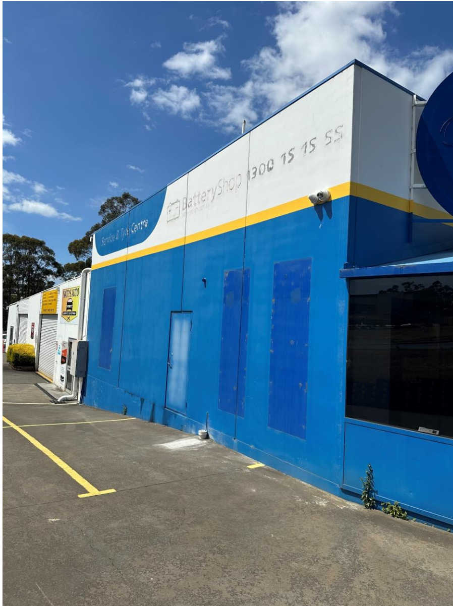
Image.3. Looking east toward the north facing elevation of the existing warehouse building at the subject site. Source: Gray Planning, taken February 2024. No image modification.
