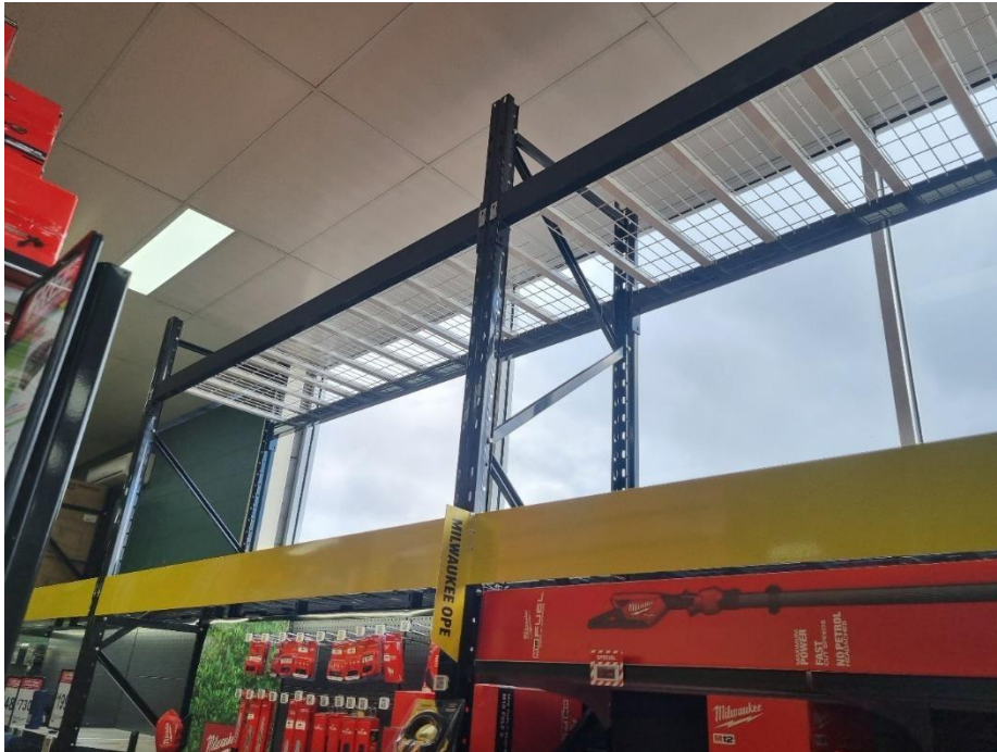
Figure 10: Upper windows through which thieves broke in.
