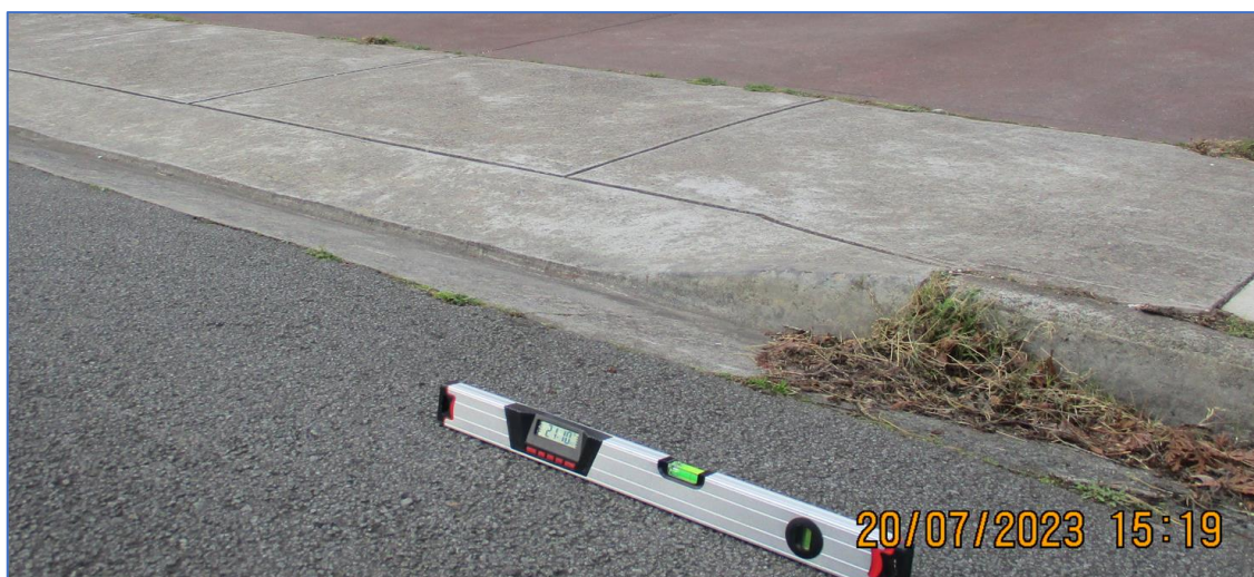
Photograph 8.7 – Vertical grade of 21 percent adjacent to car parking spaces in Howarth
