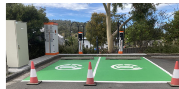
Installation of two EV charging stations in the Civic Centre car park, operated by Chargefox Pty Ltd
