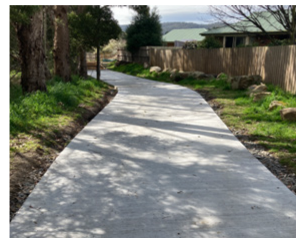
Whitewater Creek Shared Path upgrade (Summerleas Road to Southern Outlet) to 3m concrete path from Kingston Park to Summerleas Road
