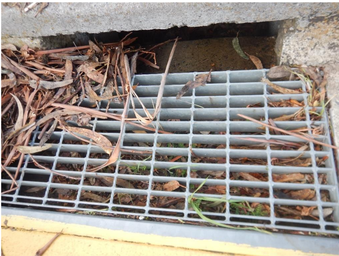
Figure 4.2 Example of Potentially Insufficient Pit Depth
