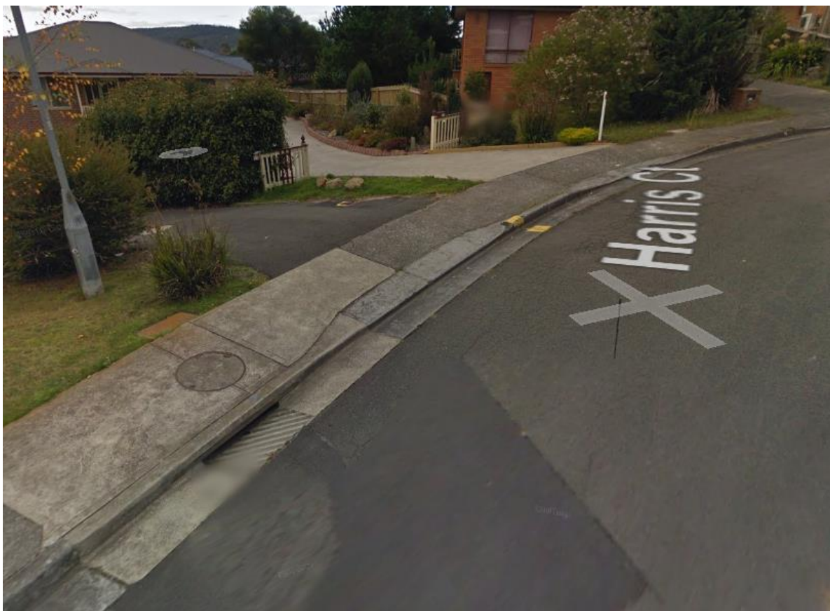
Figure 4.1 Example of Potentially Ineffective Side Entry Pit on Harris Court, Kingston
